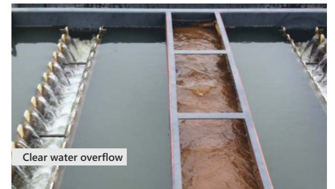
Lamella clarifier with sand filter and flocculation tank
