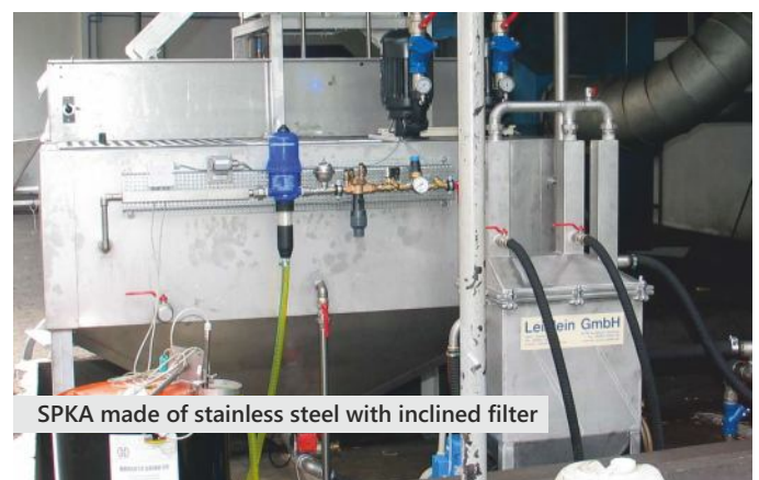
SPKA with magnetic separator and inclined filters
