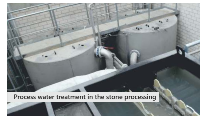
Sand filters with lamella clarifier for washing water treatment
