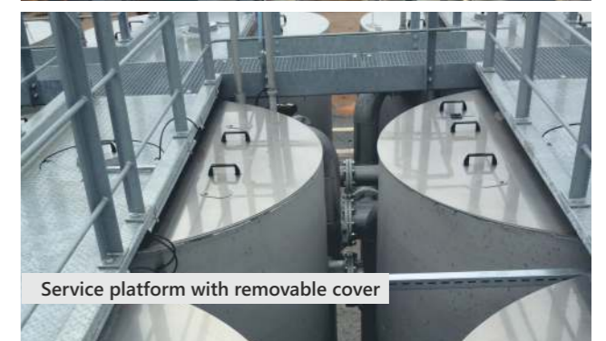
Sand filter with lamella separator and flocculation tank
