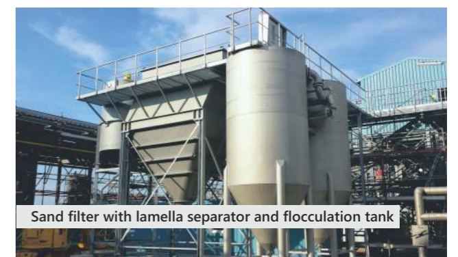
Process water treatment in the stone processing
